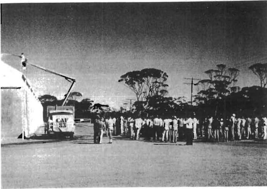
Figure 1. Detergent solution being applied to the roof of a newly sealed storage.
